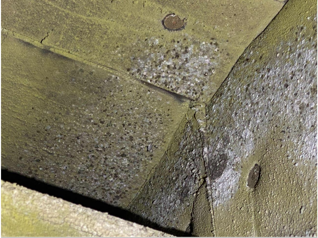
Mold in HVAC duct
