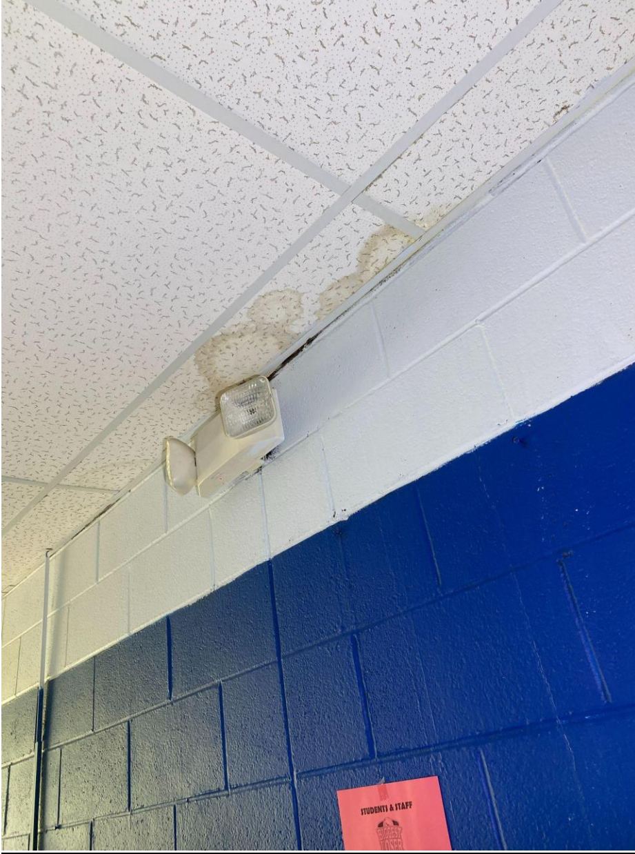
Moisture stains on ceiling tile
