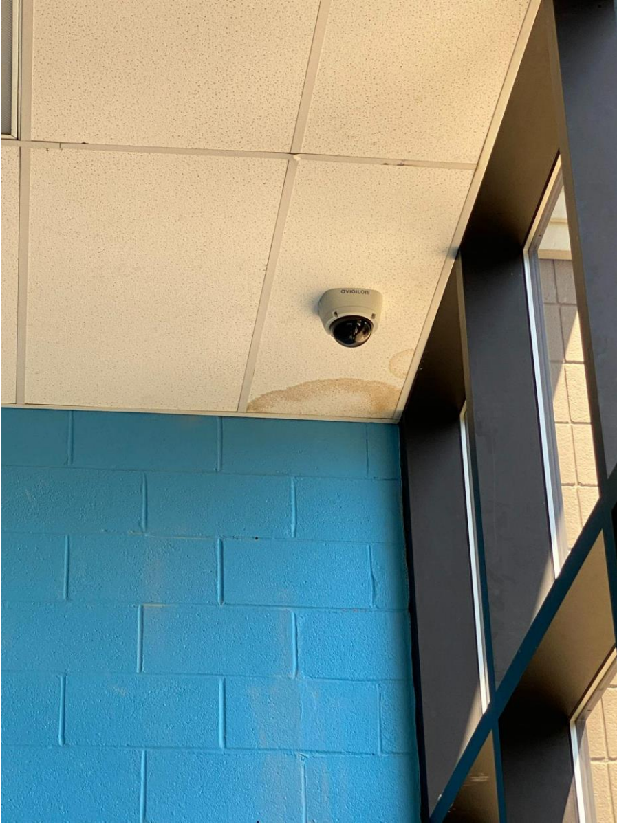
Moisture stains on ceiling tile
