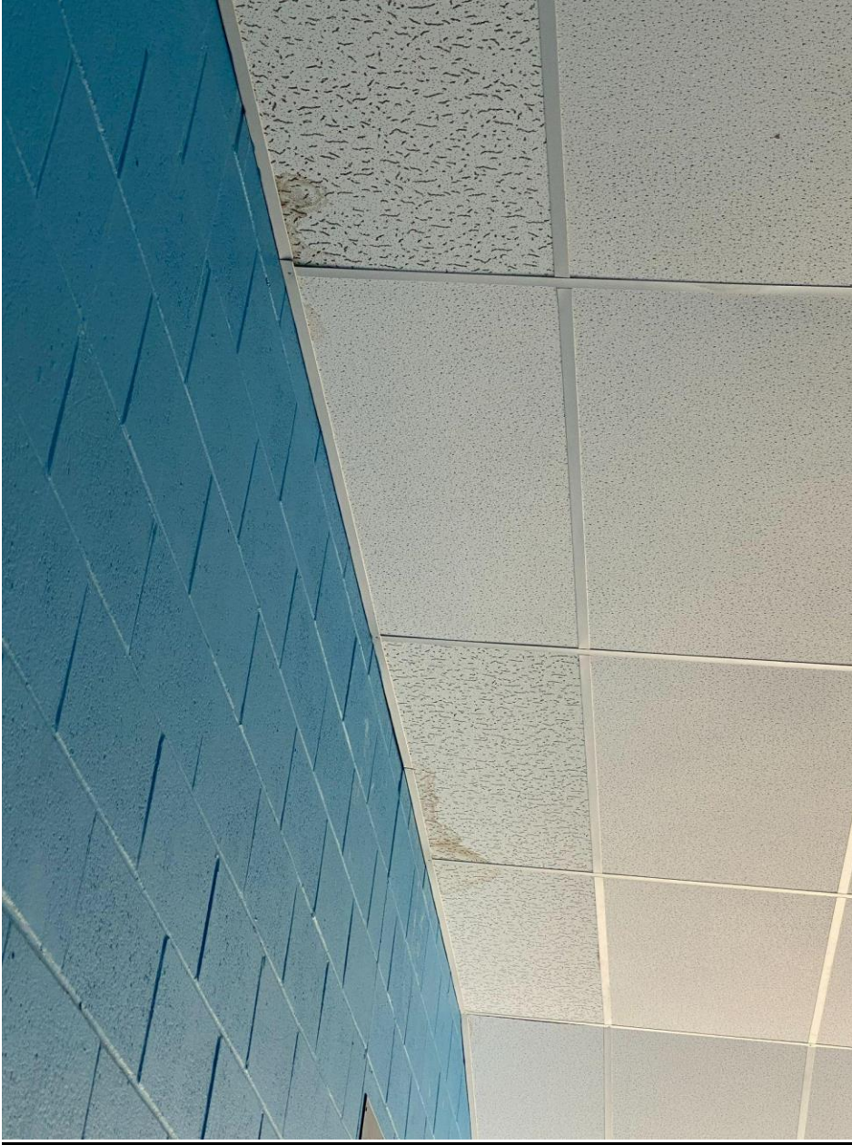
Moisture stains on ceiling tile
