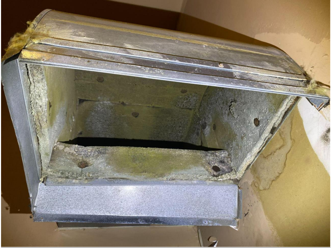
Mold in HVAC duct
