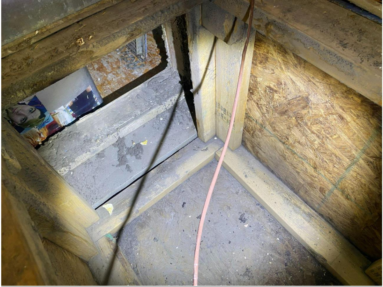
Mold in HVAC duct
